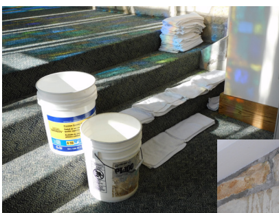
The source of longtime rain leakage in the east entryway has finally been diagnosed, and we look forward to fixing it.
