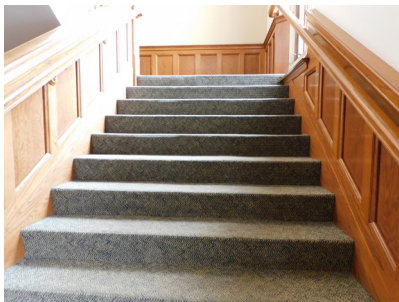
Carpeting throughout the two main staircases and Upper level is over twenty years old and showing its age. Bumps and ridges from long use are tripping hazards as well as being unsightly.
