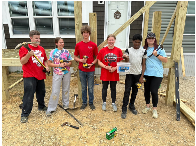
Holding the tools of their trade for the week are Tyler Goeckermann, Claire Foley, Stephen Searing, Julia Fossum, Jeremiah Finley, and Kateri Kirchner. The tools were put to good use in building a deck and accessible entrance for Ronald and Rosemary and Baby Randall.
