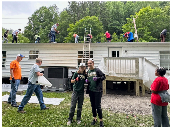
It took everyone’s help to put on a new roof at Eli and Freda’s home. The ground crew included (l to r) chaperones Tom Templeman and Kevin Slager, Calli Dahlgren and Victoria Vorpapel, and chaperone Thaurra Stallings. On the roof were (l to r) Owen Schaar, Jake Dahlgren, Ethan Antczak, Lila Thomas, Merrigan Cook, Clare Kasdorf, Sophia Searing, Jinru Granger, and Michaela Wolter.
